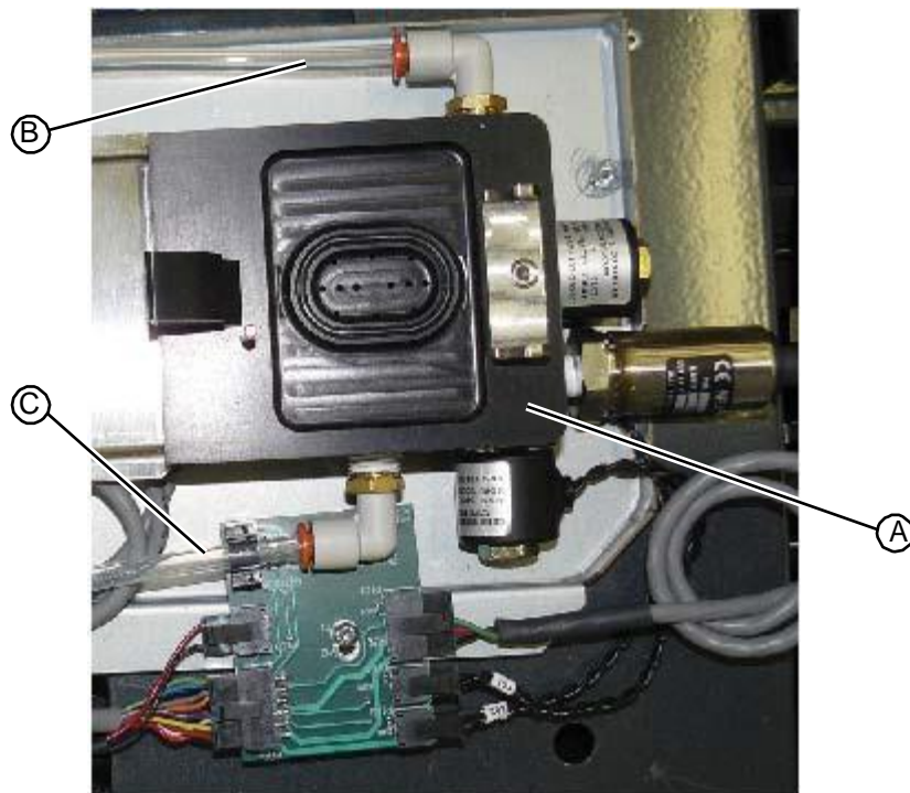
Figure 5.73: Tubing connected to the prep station manifold
