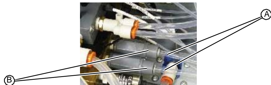
Figure 5.82: Prep station vacuum tubing connected to prep station vacuum filters
