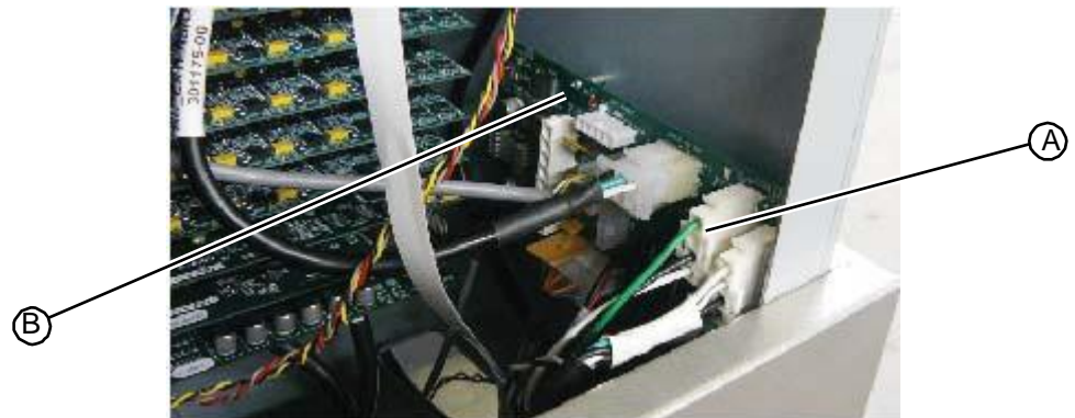
Figure 5.291: Fluid pump cable at connection P4 on the AC/DC power distribution PC board
