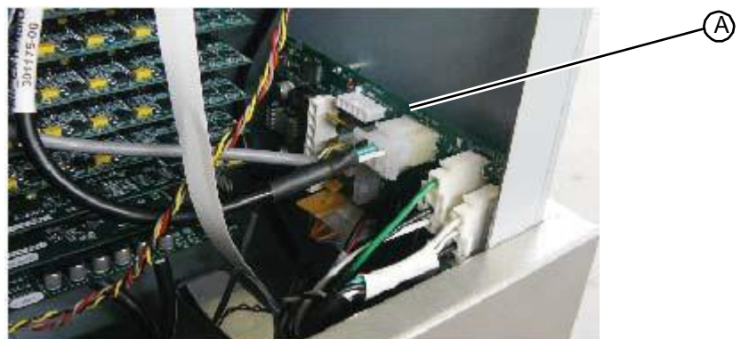
Figure 5.276: Location of AC/DC power distribution PC board in the electrical tower
