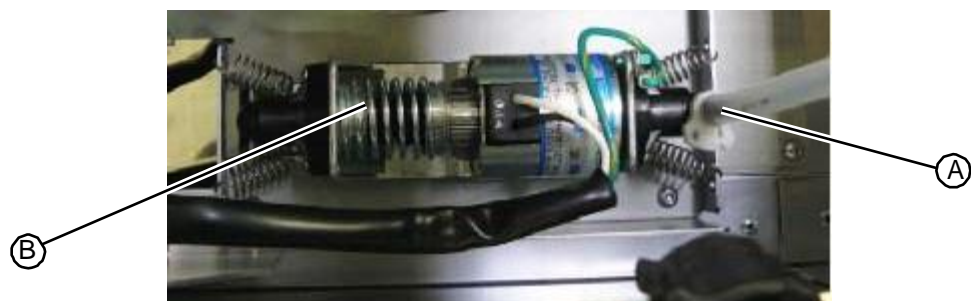
Figure 5.292: Tubing connected to the fluid pump that runs to the fluid distribution manifold
