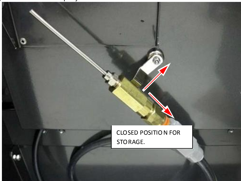
Figure 5.320: Wand Properly Positioned in Maintenance Drawer
