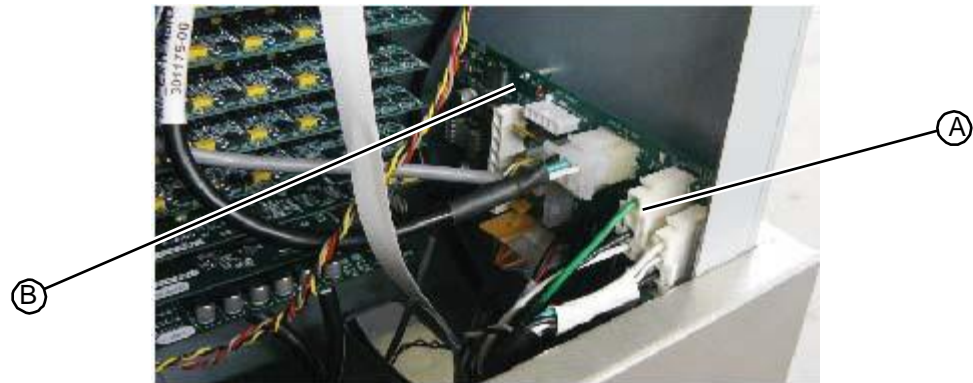
Figure 5.296: Fluid pump cable at connection P4 on the AC/DC power distribution PC board
