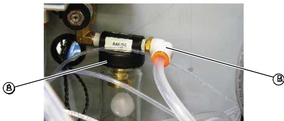
Figure 1.30: Main vacuum manifold water trap
